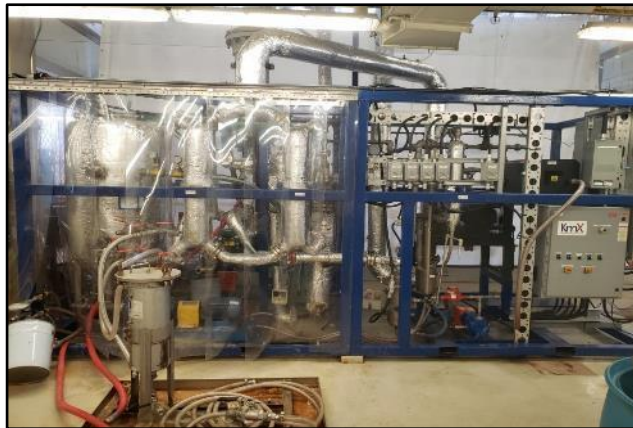
Vacuum Membrane Distillation
